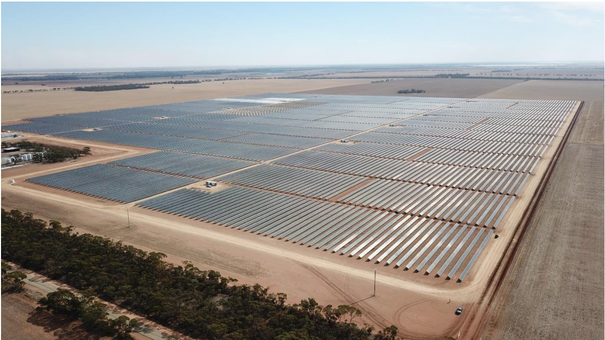
Gannawarra Solar Farm, 60MWp. Source: Wirsol Energy
